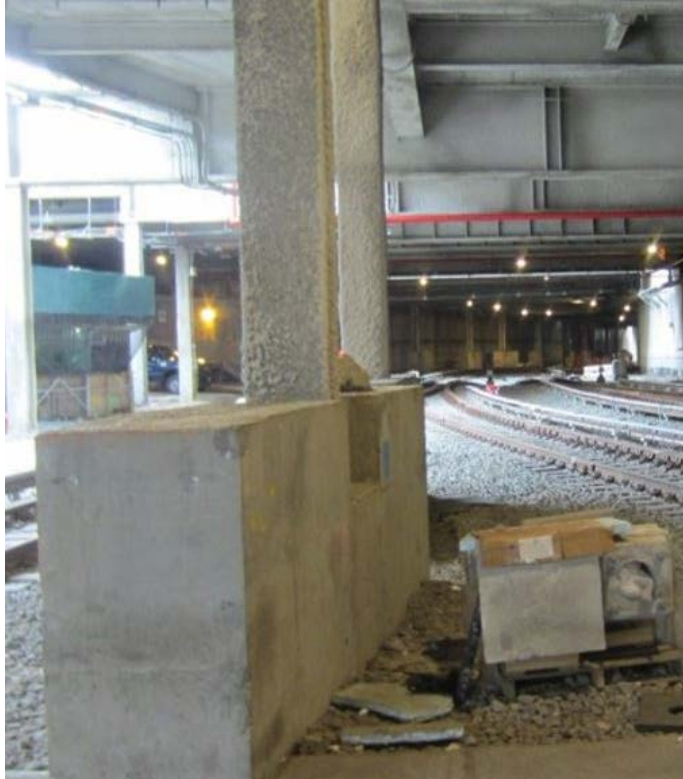
Representative conditions beneath Empire Outlets. This structural support column and others would need to be relocated to accommodate new LRT tracks.
