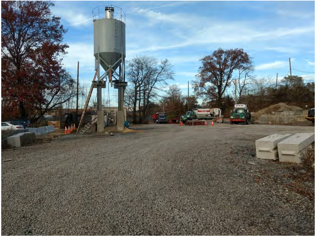
Photograph 38. Section 6, the proposed Arlington Station parcel west of South Avenue. View looking north.
