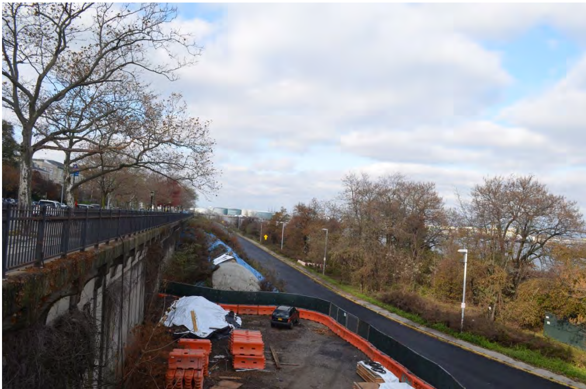
Photograph 4. Section 1, former railroad alignment under pavement in North Shore Waterfront Esplanade Park, with Richmond Terrace on left. View looking northwest.
