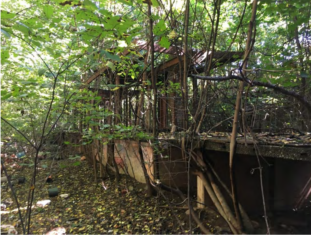
Photograph 35. Section 5, station remnants within the open cut between De Hart Avenue and Van Pelt Avenue. View looking southeast.
