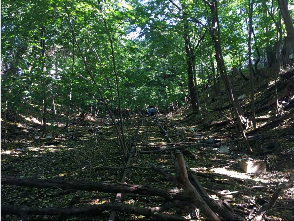
Photograph R.21. Section 5, the open cut between Van Pelt Avenue and Van Name Avenue. View looking east.
