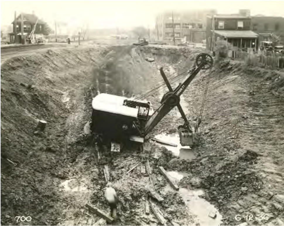
Constructing the open cut and the Lake Avenue station in 1936. Courtesy Gary Owens, http://www.gretschviking.net/GOSIRTNorthShore2.htm .
