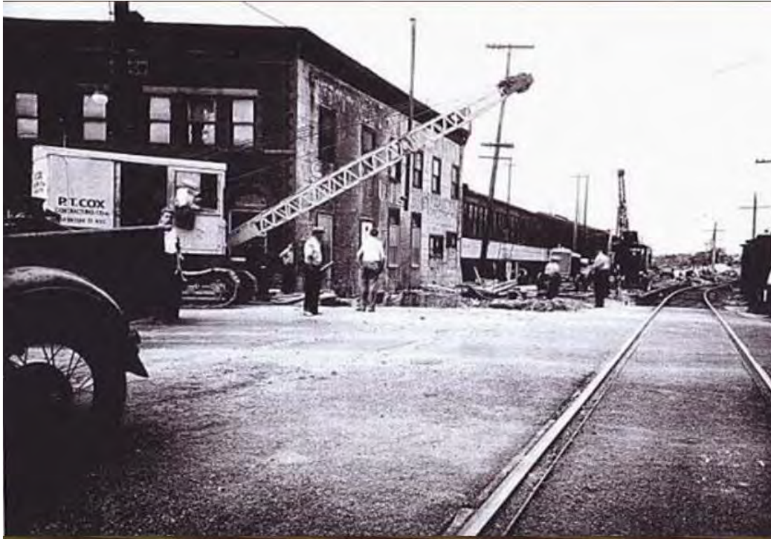
Richmond Terrace, excavating for the viaduct on left in 1935. Courtesy Gary Owens, http://www.gretschviking.net/GOSIRTNorthShore.htm .
