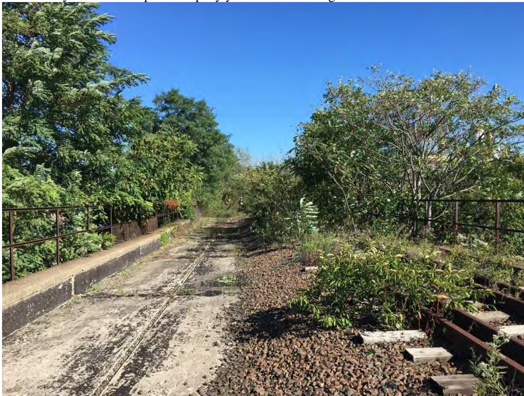
Photograph R.12. Section 4, conditions on top of the viaduct near the Port Richmond Wastewater Pollution Control Plant. View looking east.
