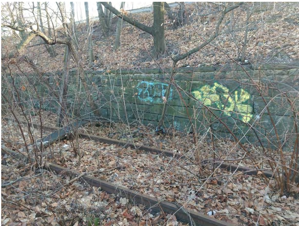
Photograph 14. Section 2, former railroad tracks and stone retaining wall at Sailors' Snug Harbor, with Richmond Terrace in the background. View looking southeast.
