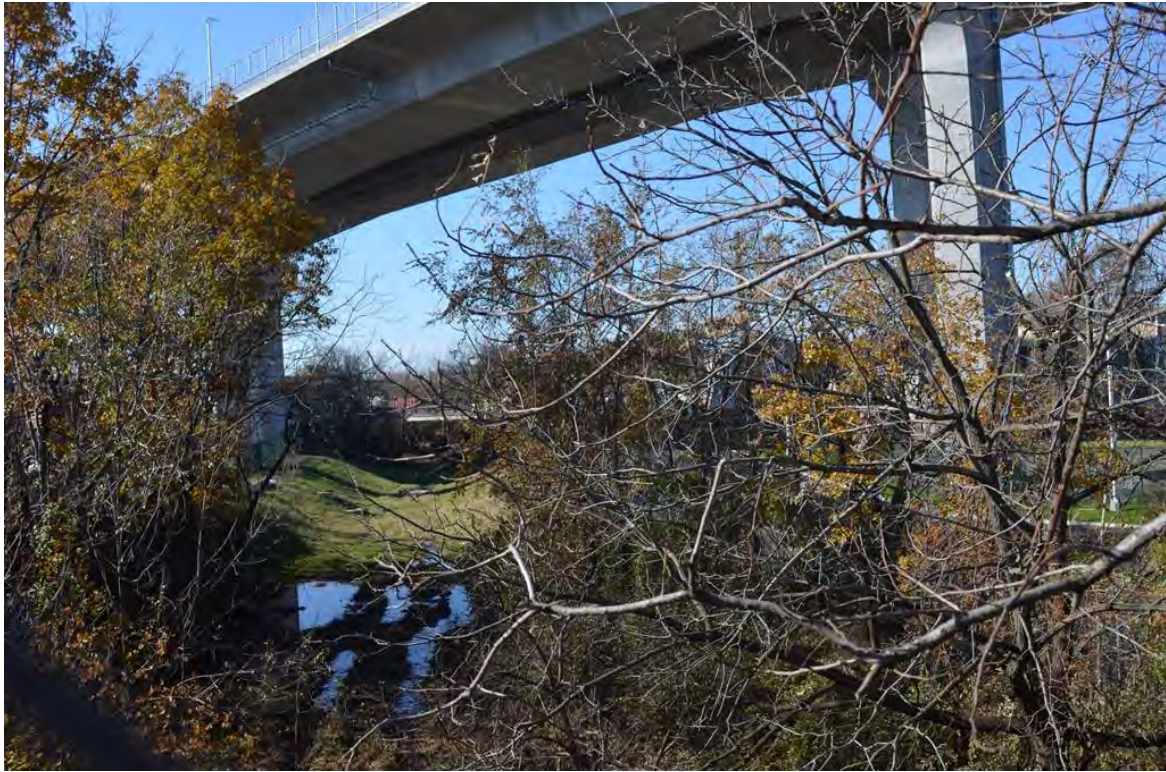
Photograph R.18. Section 5, remains of the open cut filled with water under the Bayonne Bridge approach. View looking southwest.
