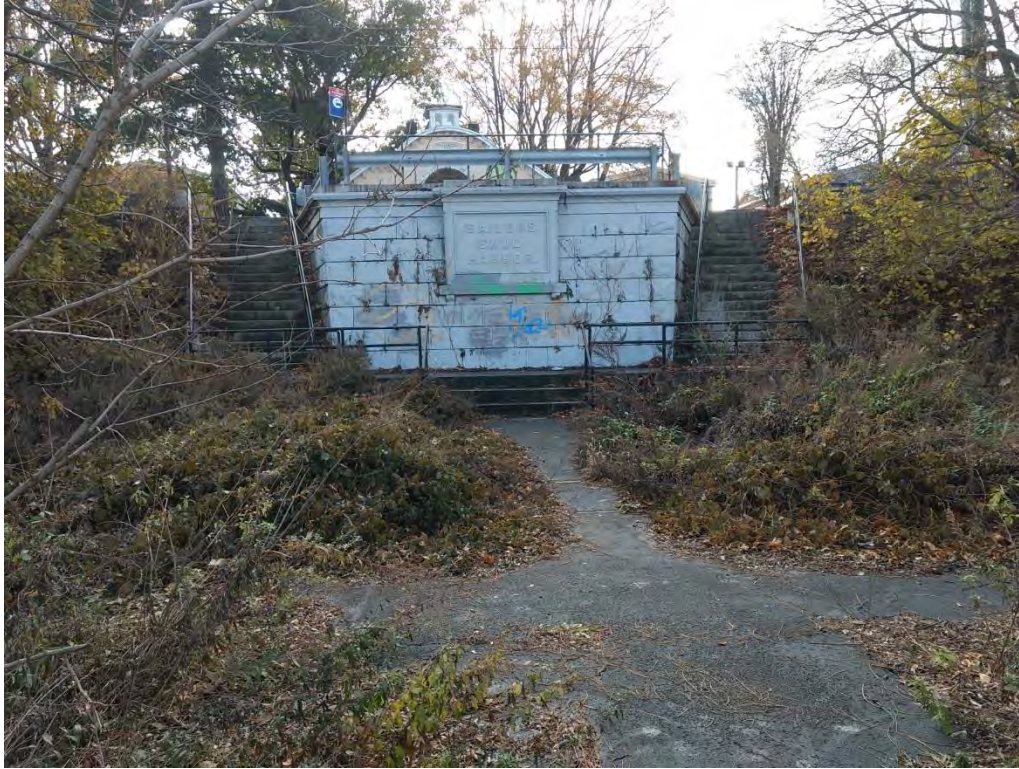
Photograph 2.23. Sailors' Snug Harbor historic viewing platform on north side of Richmond Terrace. View looking south.
