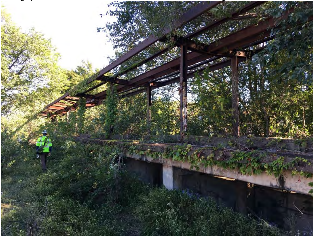
Photograph R.16. Section 4, former station remains on top of the viaduct near Sharpe Avenue. View looking southeast.
