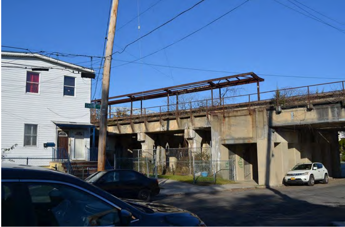
Photograph R.17. Section 4, former station remnants on top of the viaduct near Sharpe Avenue. View looking northwest.
