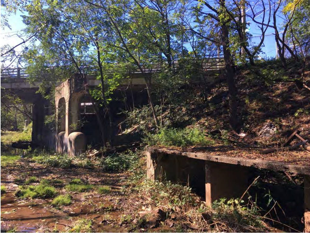
Photograph 33. Section 5, the open cut near Morningstar Road, with station remnants. View looking west.
