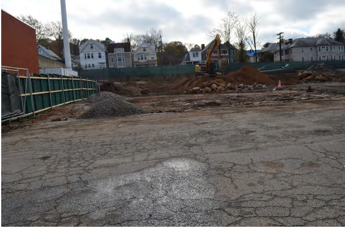
Photograph 2.7. Proposed staging area on the south side of Richmond Terrace near Franklin Avenue, with houses in the background on Van Buren Street. View looking south.
