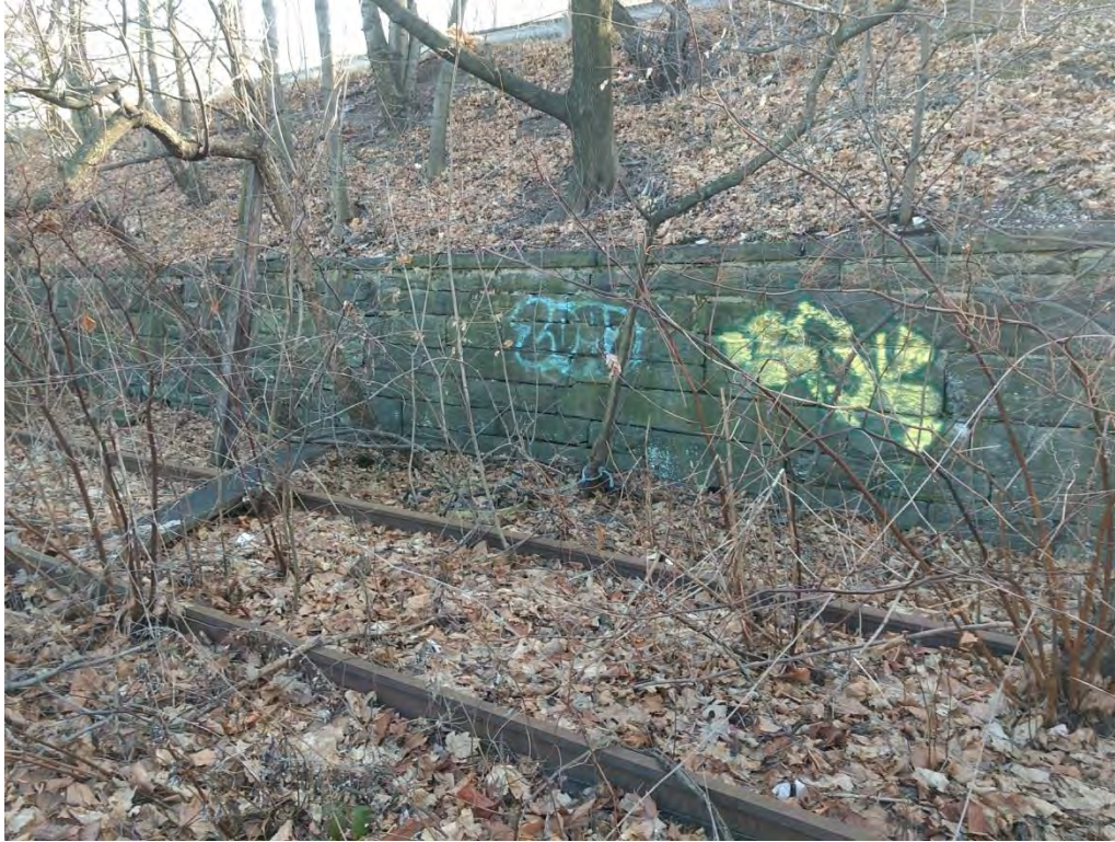
Photograph 2.27. Former railroad tracks and stone retaining wall at Sailors' Snug Harbor, with Richmond Terrace in the background. View looking southwest.
