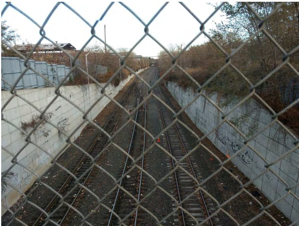
Photograph R.24. Section 6, active tracks at the South Avenue overpass. View looking east.
