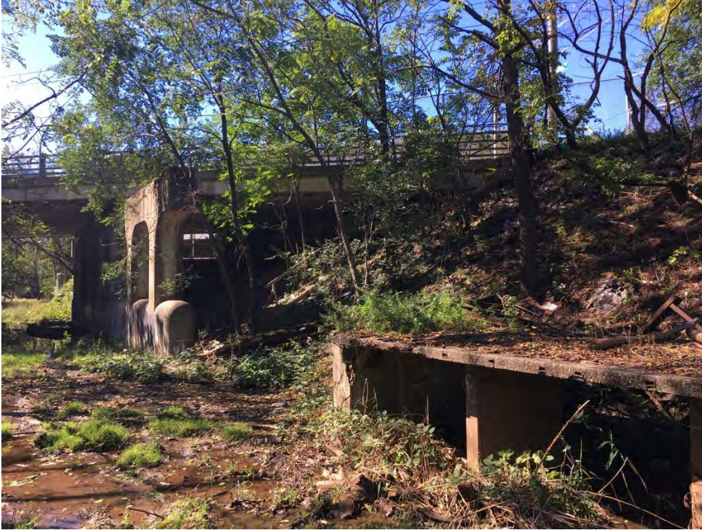
Photograph R.19. Section 4, the open cut near Morningstar Road, with station remnants. View looking west.
