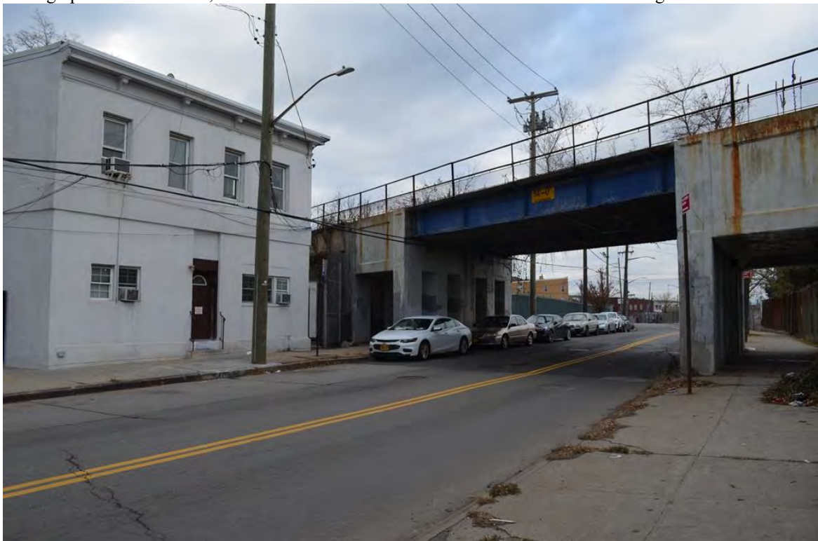
Photograph R.14. Section 4, the viaduct crossing at Richmond Terrace. View looking northwest.
