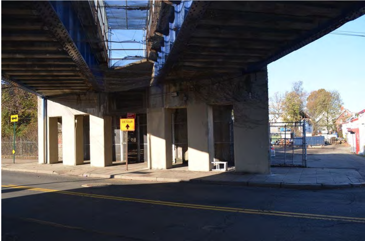
Photograph 29. Section 4, detail of the viaduct underside crossing Port Richmond Avenue. View looking west.
