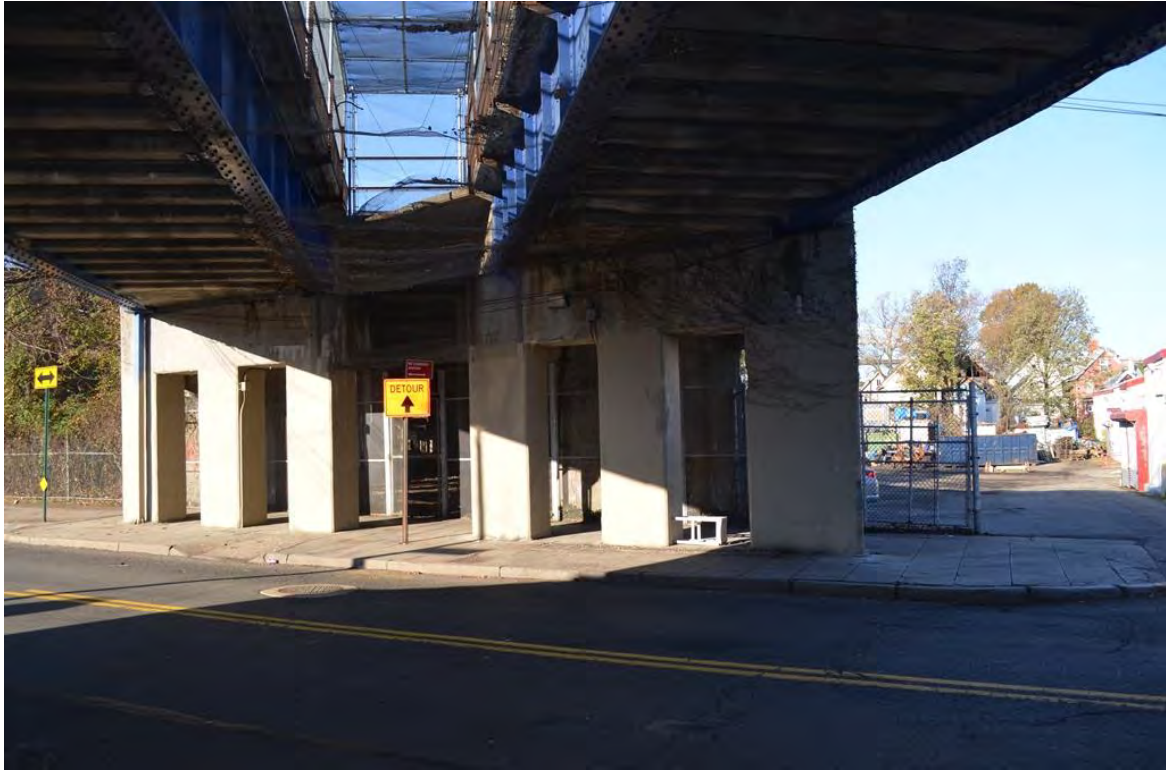
Photograph R.15. Section 4, detail of the viaduct underside crossing Port Richmond Avenue. View looking west.
