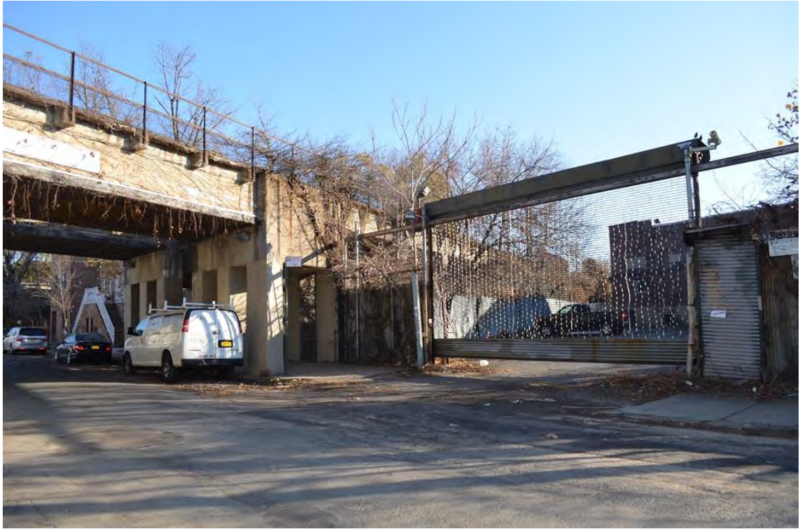
Photograph 4.18. Maple Avenue south of the viaduct, rear of 108 Port Richmond Avenue. View looking northeast.
