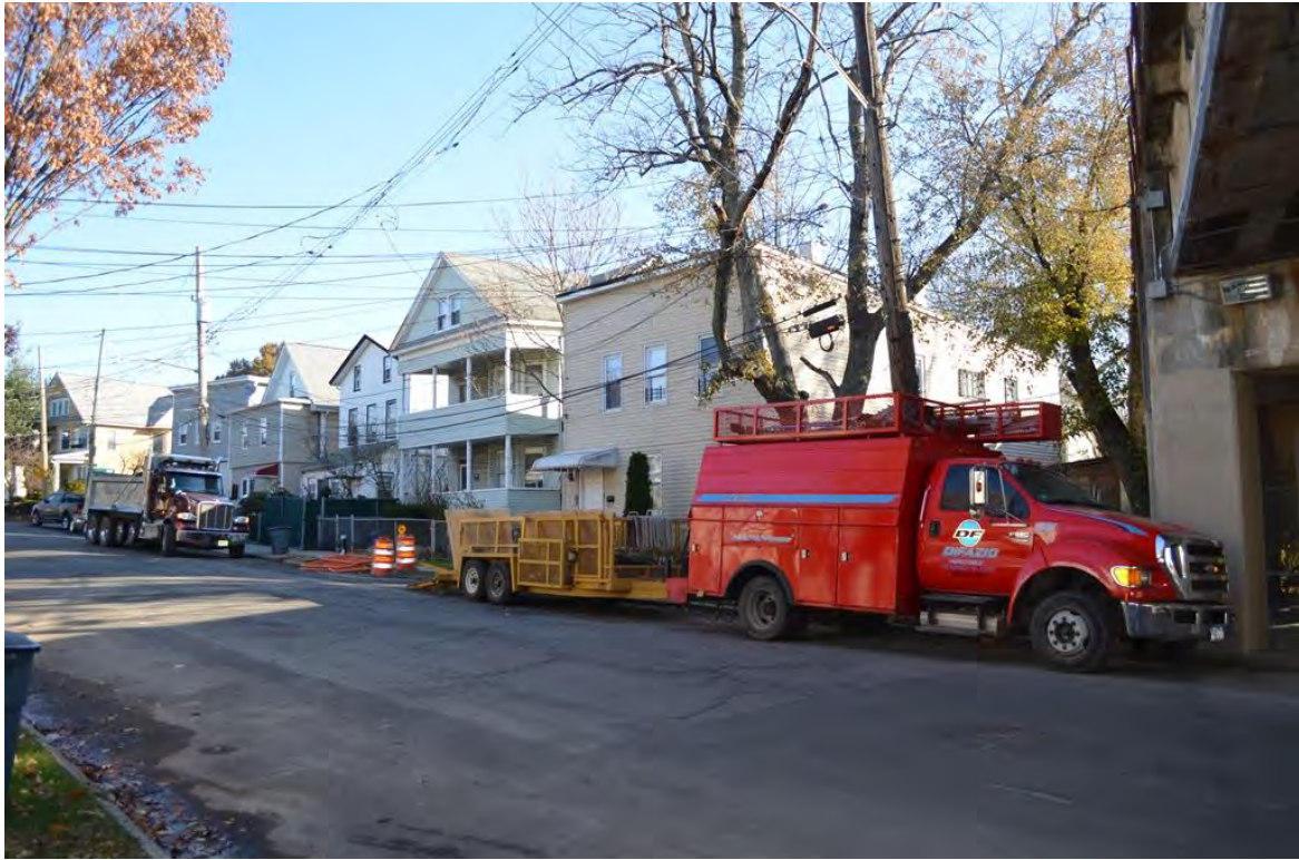
Photograph 4.26. Faber Street north of the viaduct. From right: 55, 51, 47, and 45 Faber Street (Block 1074, Lots 15, 18, 20, and 22). View looking northeast.
