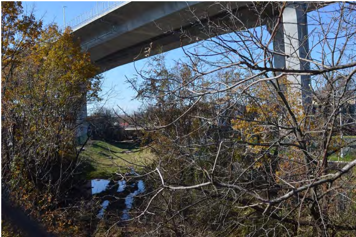
Photograph 32. Section 5, remains of the open cut filled with water under the Bayonne Bridge approach. View looking southwest.
