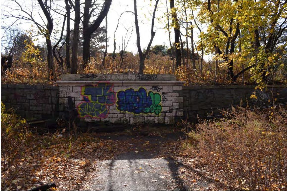
Photograph 15. Section 2, the stone retaining wall at Sailors' Snug Harbor, at the base of the paved paths. View looking south.
