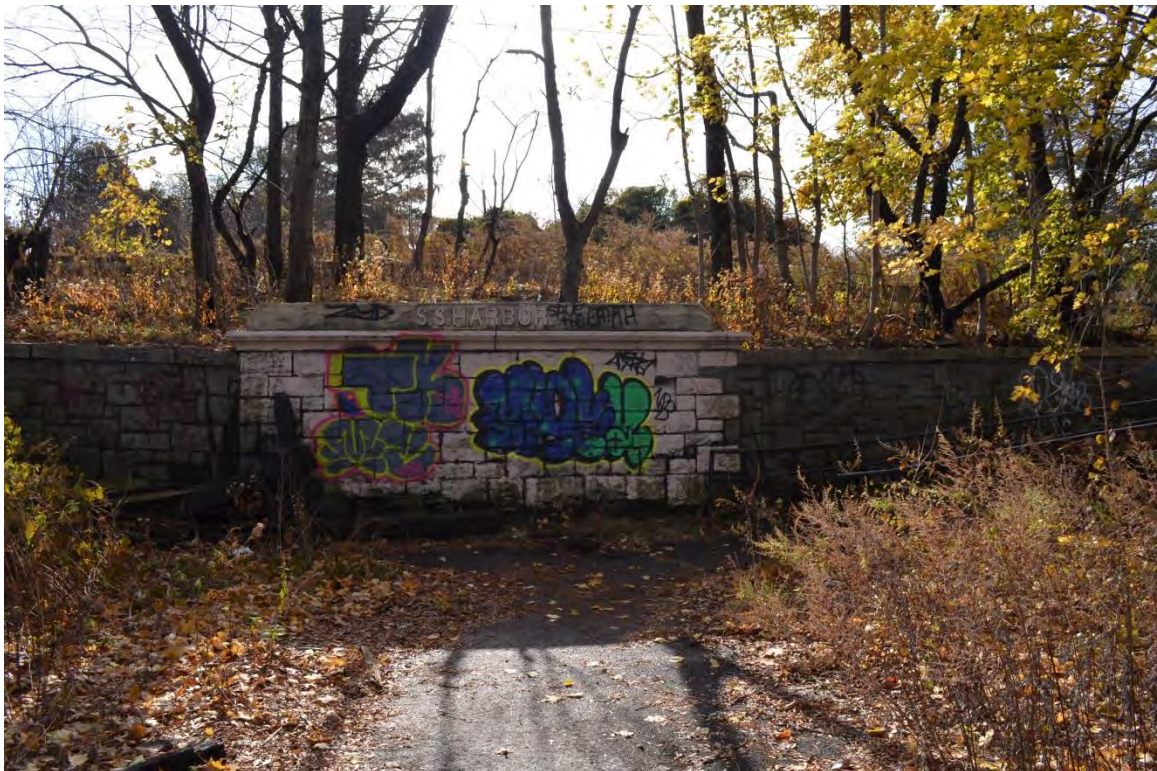
Photograph 2.28. Stone retaining wall at Sailors' Snug Harbor, at base of paved paths. View looking south.
